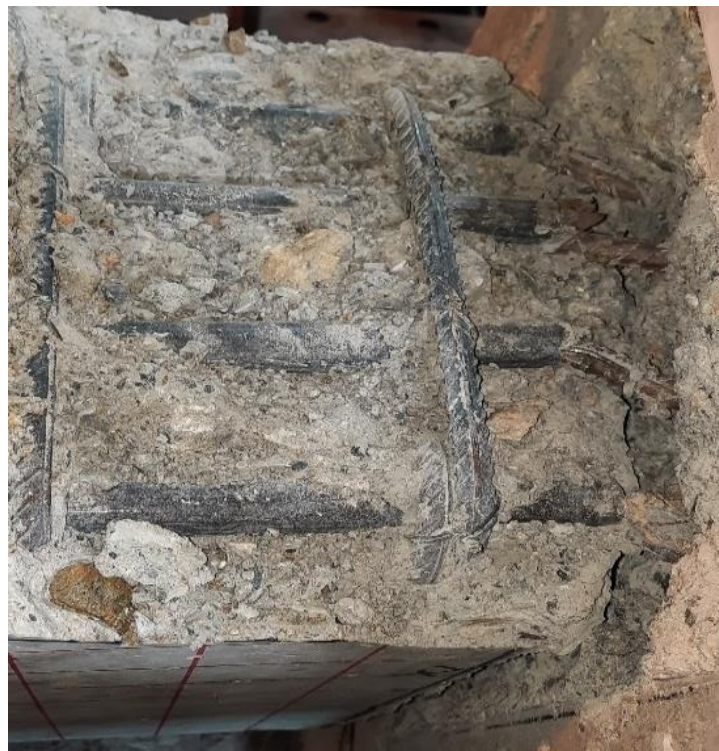
Fig. 9. Buckling state of the longitudinal rebar in specimen No. 2 with steel tube. Note that the rebar buckling start in the cover of stub column.
