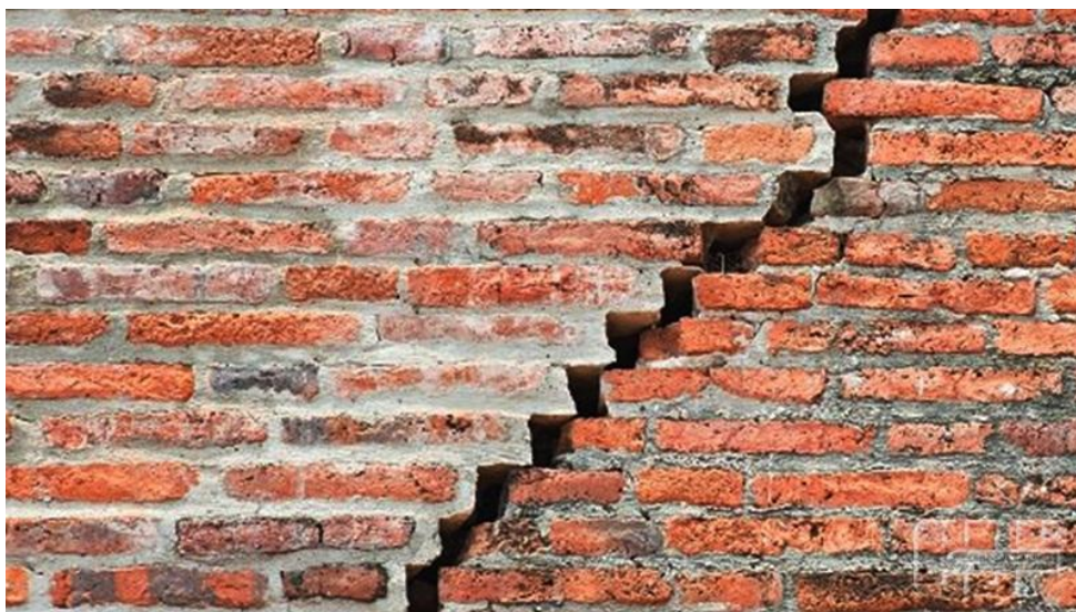
Fig. 1. Masonry shear failure source: cendana news [39].
