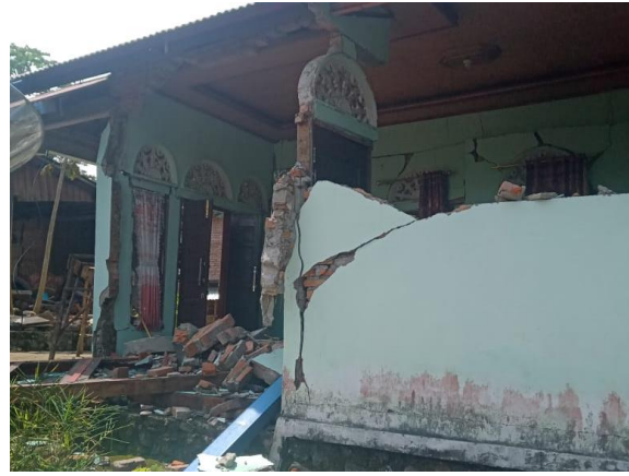
Fig. 2. Masonry flexural failure.
