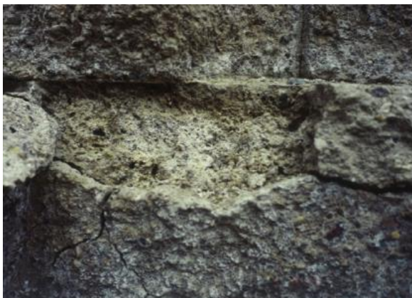
(a) The appearance of precast concrete as a retaining wall under thaumasite sulfate attack
