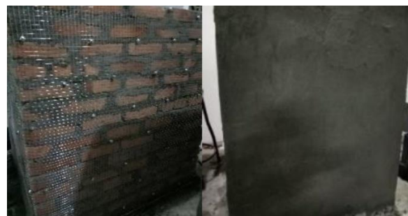
Fig. 17. Ferrocement Layers on masonry wall. Left: Wire mesh and Right: Concrete coating. [13].
