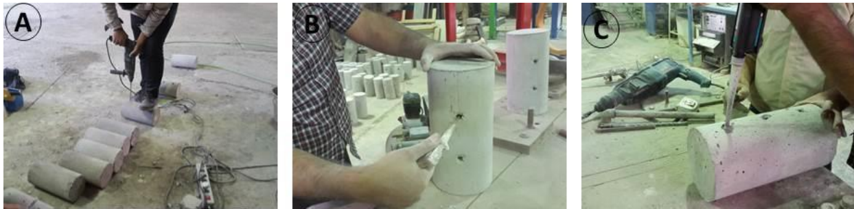
Fig. 4. Displays the process of rebar planting inside the concrete, a) Drilling the holes, b) cleaning the holes before casting glue, and c) casting the glue.
